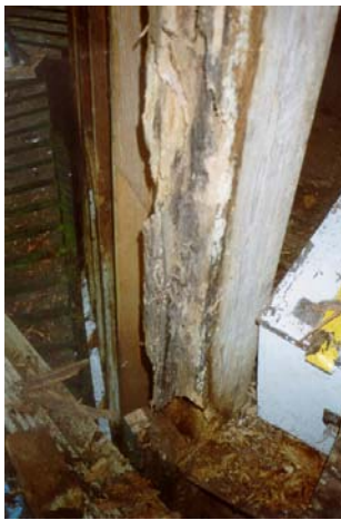
Timber failure on cant post
