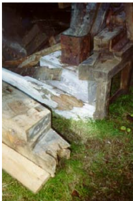
Junction of the Breast Beam and Shear showing failed dovetail
