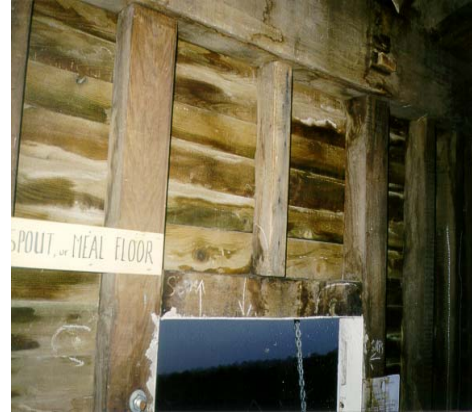
Sodden and failed weatherboarding
